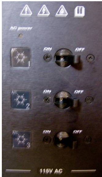
Fwd air conditioning unit
