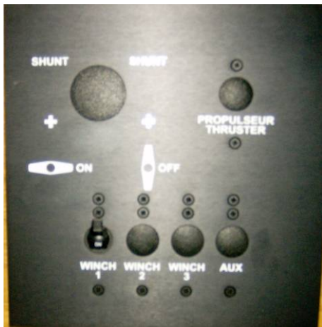
electric winch breaker
