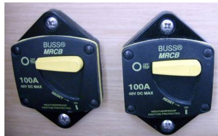
Breakers have tripped.
