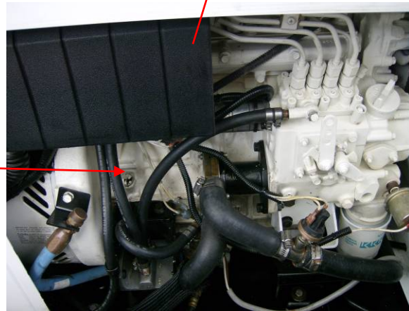
Inside the front panel of the generator
