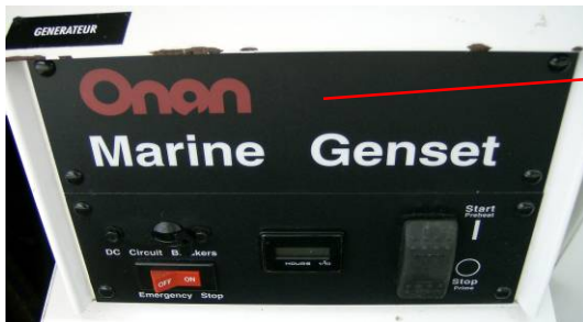
Main breakers for the generator
