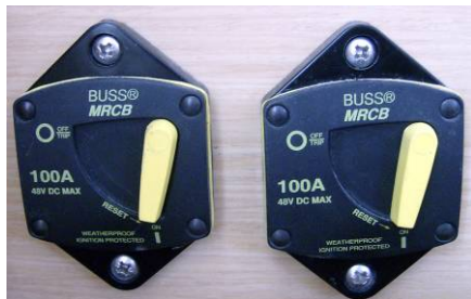
Breakers are on
