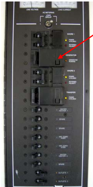
Shore power/generator selector switches
