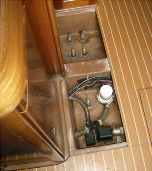
The float switch for the primary bilge pump is located near the galley
